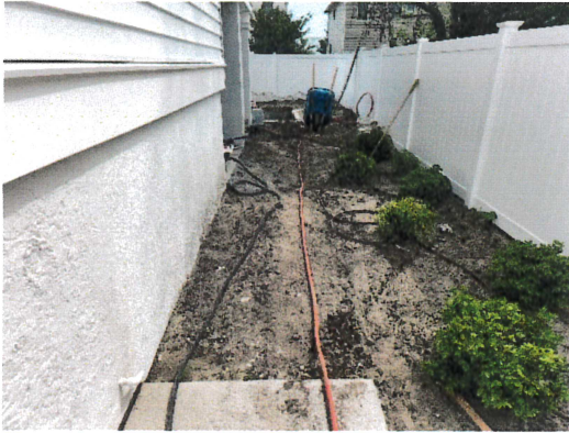
Landscaping is incomplete
