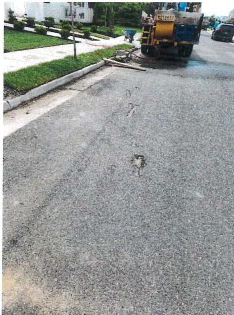
Damage done to the street, debris and dirt
