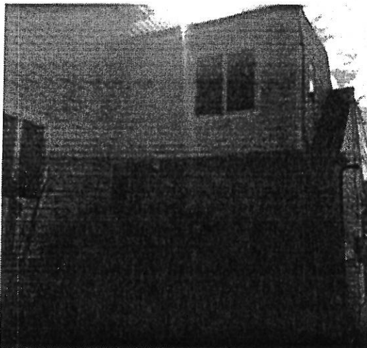
A/C Units & Generator 4-23-15
